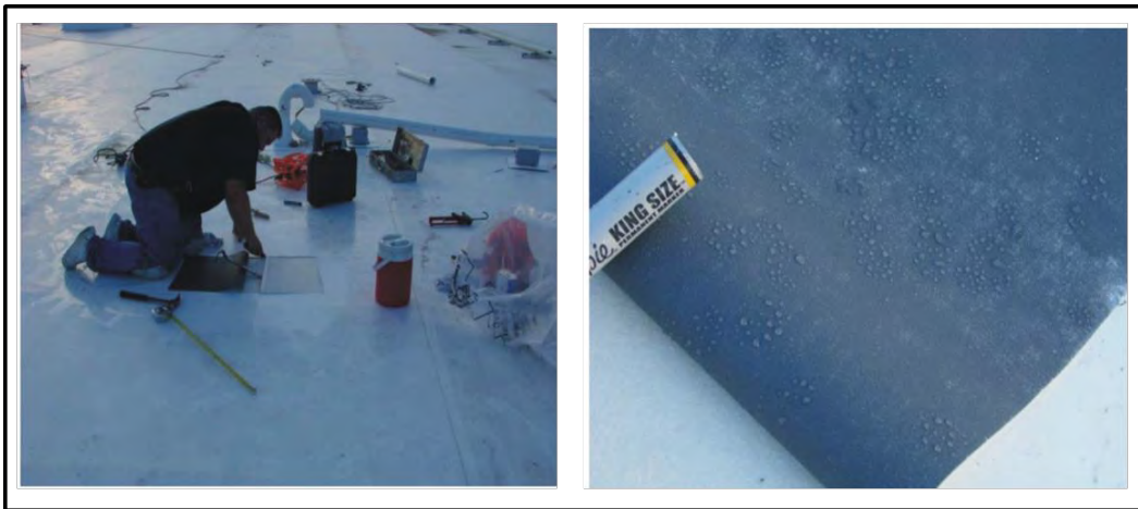
Figure 17: Condensation below the roof membrane
