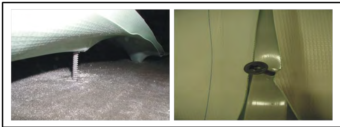
Figure 4: Fastener pullout from the steel deck
