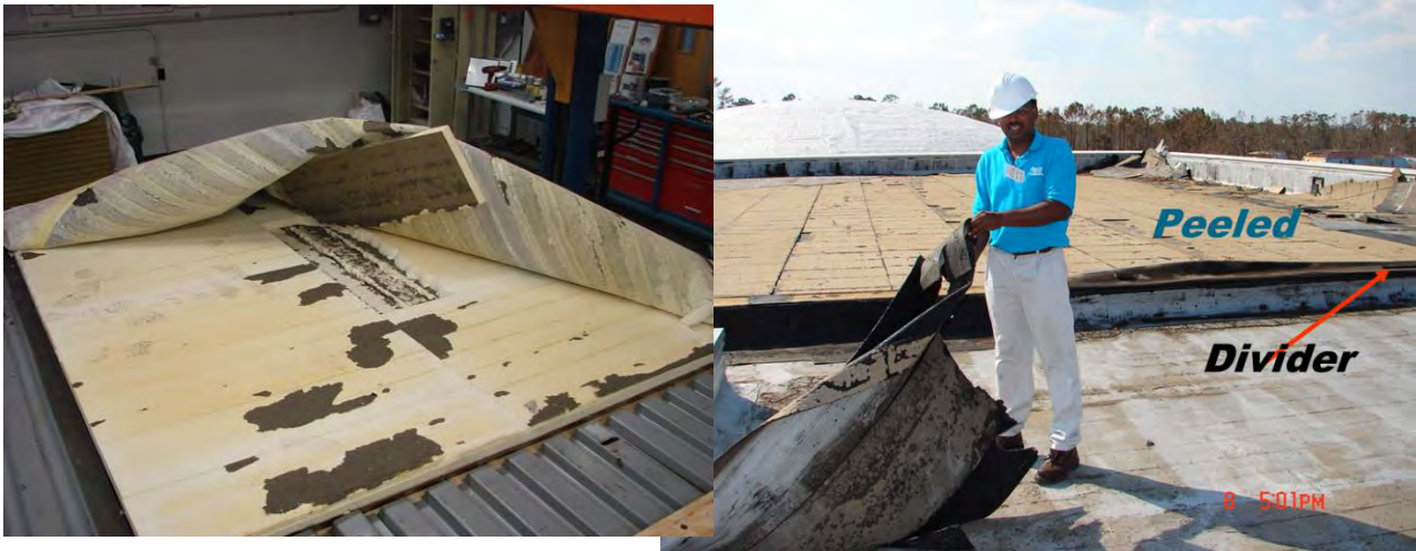
Figure 10: Facer delamination failure
